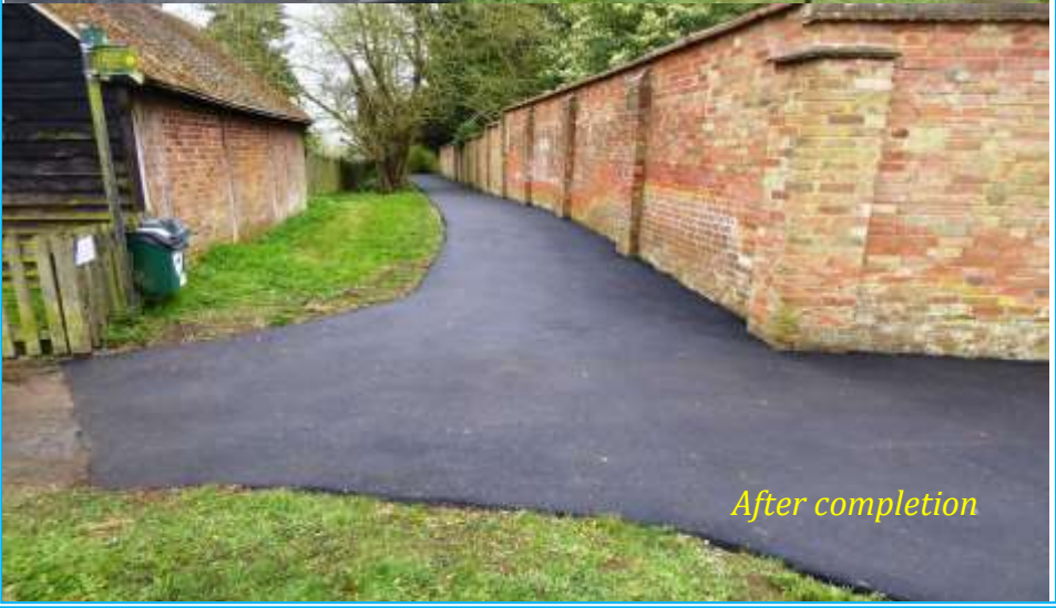
Friendly workmen from Edwards Surfacing Ltd. of Great Horwood at work on 25th April
